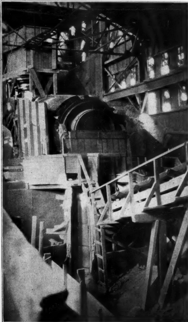
Primary Scalping Screen with Secondary Crusher Below
